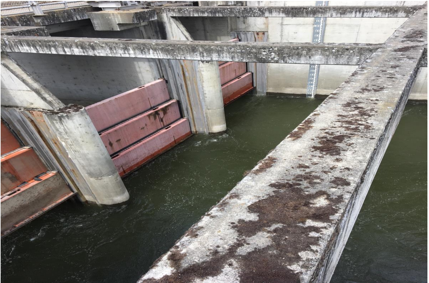
Junction pool weirs dragging from high tailwater. Limits adjusted to clear surface.
